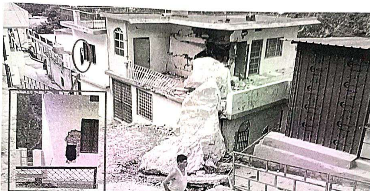
Damaged (Fully/Partially) Residential Buildings
