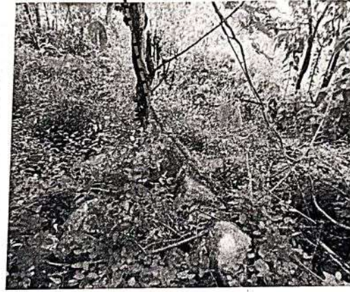
Evidence of old Debris/Rock Fall
