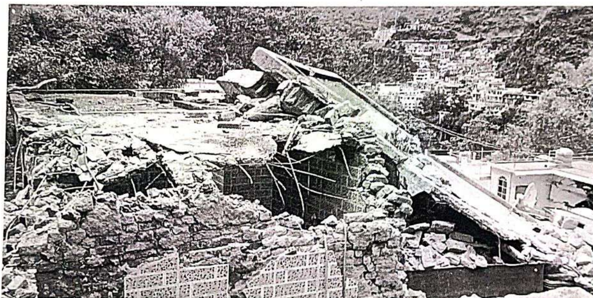
Damaged Public Toilet
